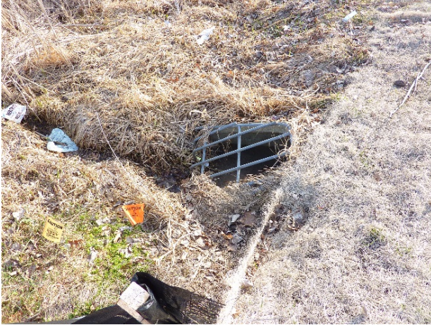
Figure 7. FES with debris
