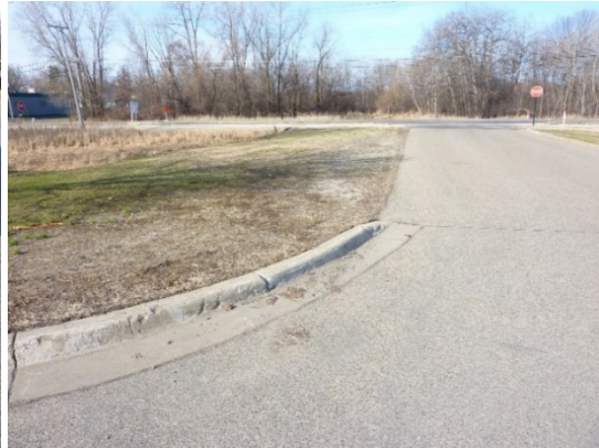
Figure 11. Crumbling curb along driveway facing Central Ave
