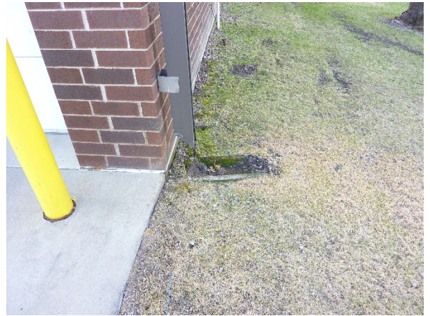
Figure 8. Concrete splash pads crumbling at base of downspout
