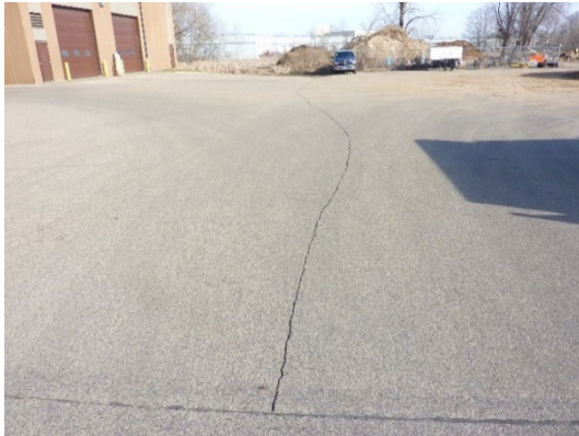
Figure 10. Large pavement crack east of storage building
