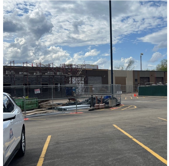
Main building garage connected to the North garage to form new cold storage space—May 3, 2024.
